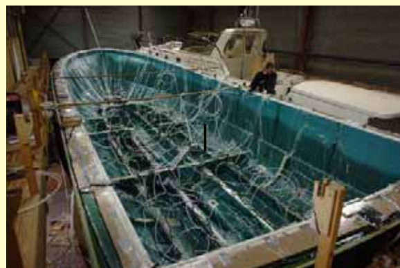
Infusion of a 42' hull and inner stiffeners in a single shot. Images courtesy of Jachtbouw Zevenhuizen BV, Franeker, The Netherlands.
